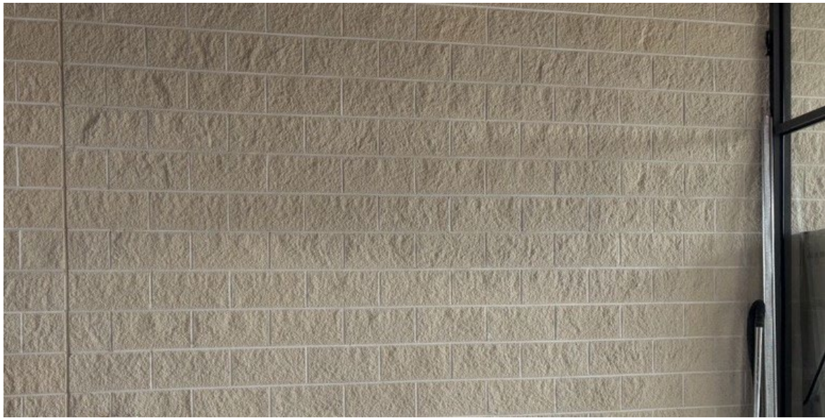
Figure 3: Block Work Finish (rough surface)
