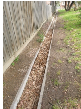
Inadequate drainage and kerbing at the southern boundary of the reserve
