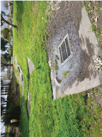
Inflow drainage pit - retarding basin
